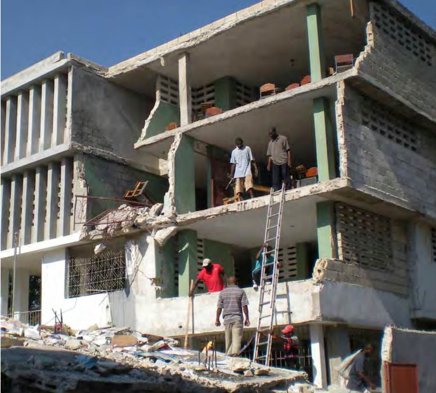
The damage to College Catherine Flon in Carrefour, Haiti.
