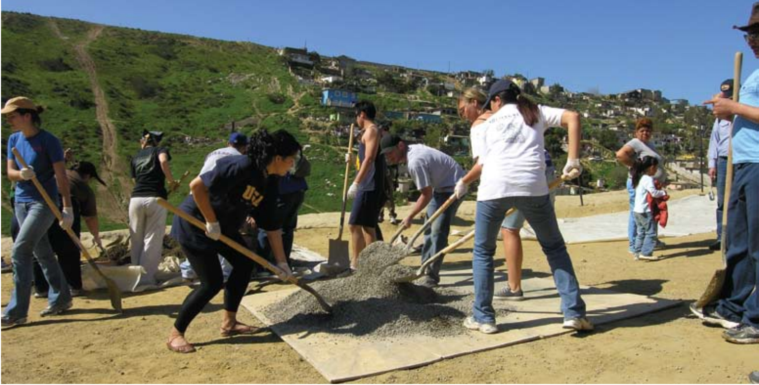
Students from UCSD Urban Studies and Planning Program's Student Club continue working on the pervious pavers on the Colonia San Bernardo elementary school playground.
