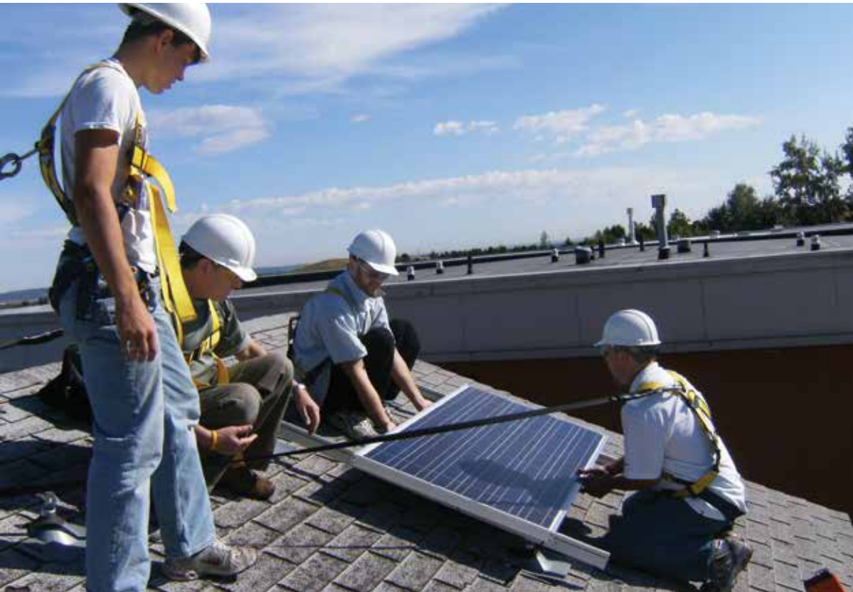
Red Rocks Community College students installing solar panels in the roof lab in Lakewood, Colorado.
