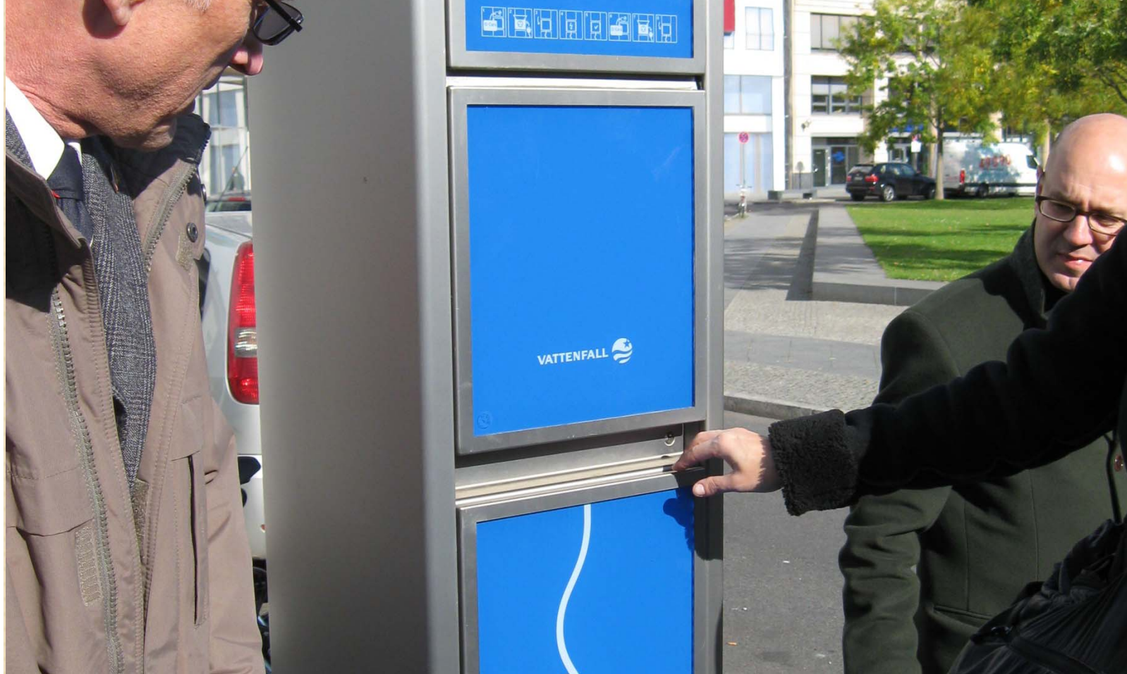
Electric Car Charging Station
